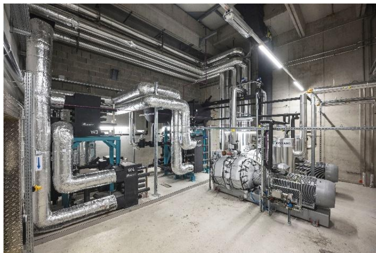
Figure 8: Installed heat pump at MPREIS premises.
